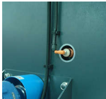
Picture 4-28: Level Switch on Mixing Tank
