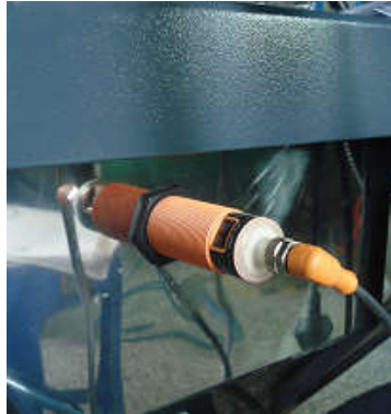
Picture 4-29: Level Switch on storage Tank
