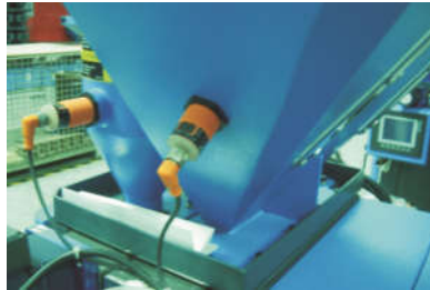
Picture 4-27: Level Switch on Hopper
